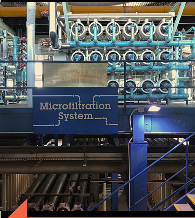
Microfiltration system at Bedok NEWater Factory, Singapore
